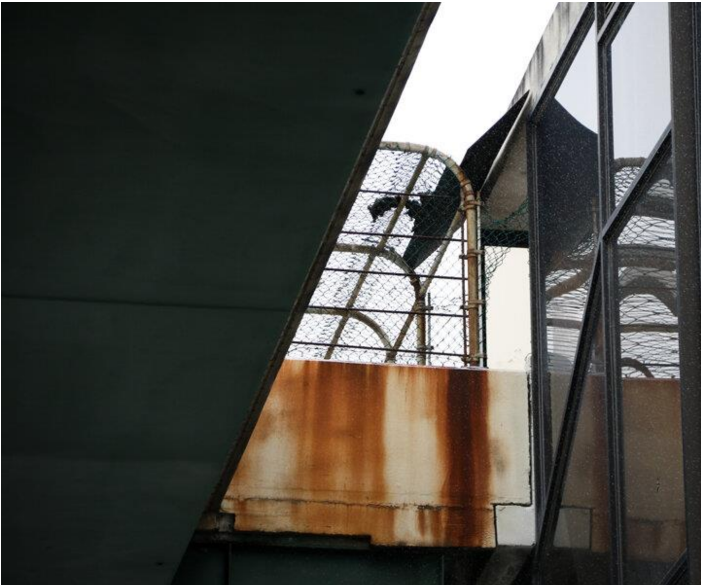
- Detail of the fencing surrounding the walkway alongside the highway exit ramp.
