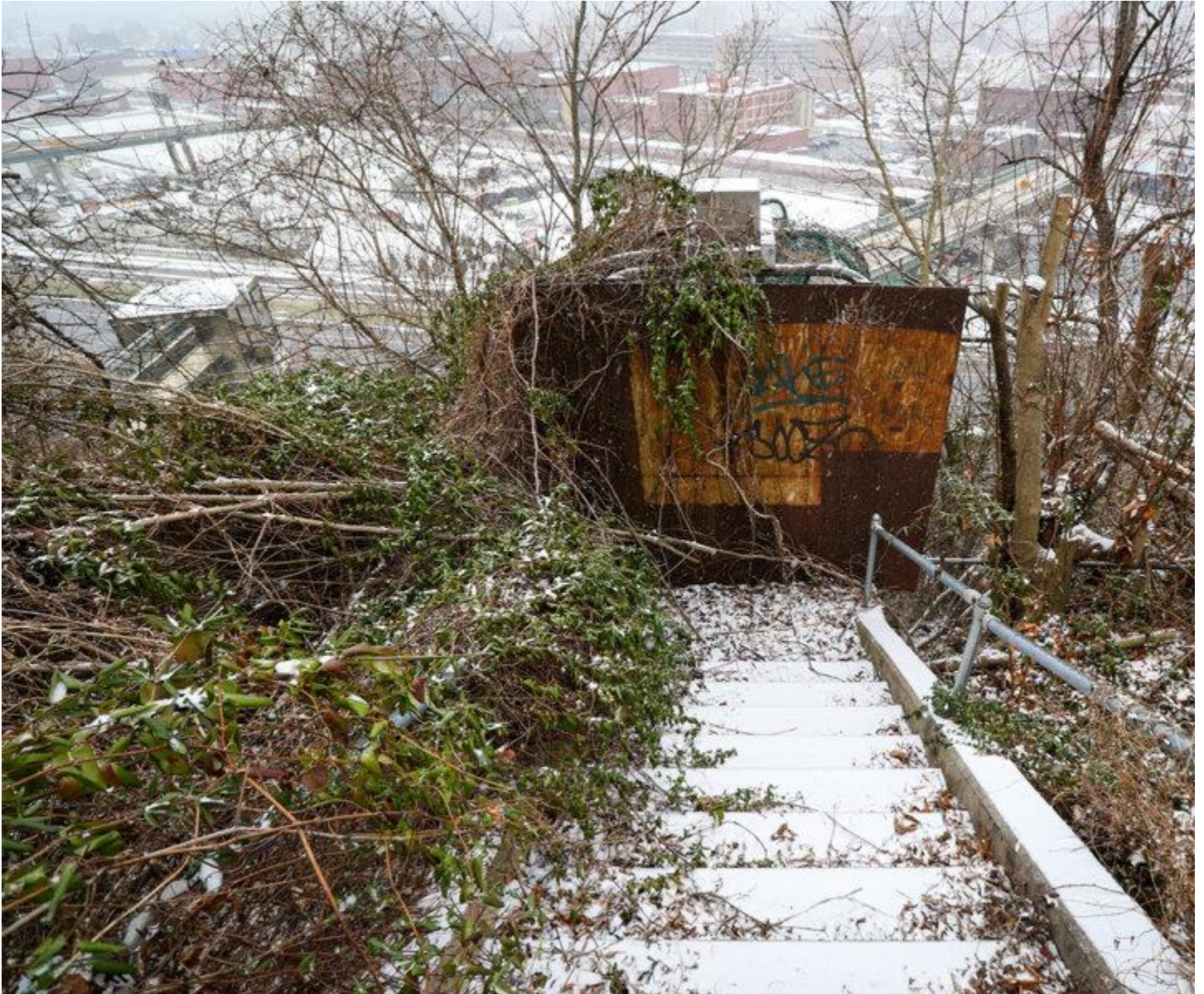
- Blocked access to the rest of the walkway and towers.
