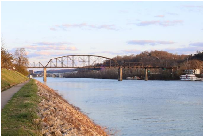
The Kanawha Bridge is an abandoned railway bridge over the Kanawha River in Charleston, West Virginia. The bridge is of a Parker through-truss design. The bridge is located east of the Patrick Street Bridge and is now named the "Travis L. Castle Railroad Trestle."
