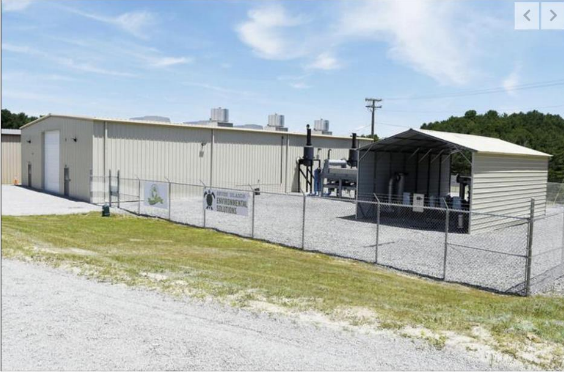
The new clean energy facility at the Raleigh County Landfill houses two 20 cylinder Caterpillar engines that convert methane from the landfill and converts to electricity on the local grid. The facility cost $5 million and had major support from Seven Islands Environmental Solutions. (Chris Jackson/The Register-Herald)
