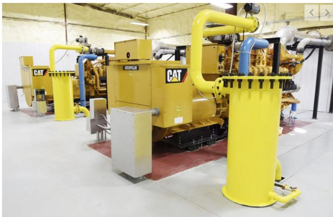
The two generators, which are 20 cylinder Caterpillar engines, convert methane captured from their landfill, cool it then converts it to electricity and puts into the local power grid. They can convert 600-700 standard cubic feet per minute of methane gas, said Raleigh County Landfill Executive Director James Allen. (Chris Jackson/The Register-Herald)
