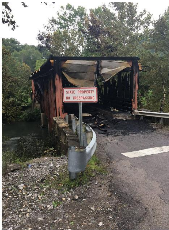
Most of the roof and walls of the 161-year-old Carrollton Covered Bridge went up in smoke during a fire Thursday night. Photos courtesy W.Va. Dept. of Transportation
