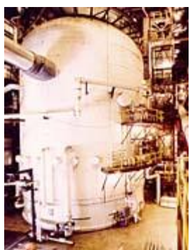
The Ohio Power Company built this advanced pressurized fluidized bed boiler near the town of Brilliant, OH, as part of a joint project with the U.S. Department of Energy.
